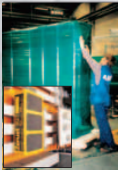
An electrical control cabinet protected inside by ZERUST® Vapor Capsules and protected outside with combination ZERUST® Multimetal/Anti-Static film.
